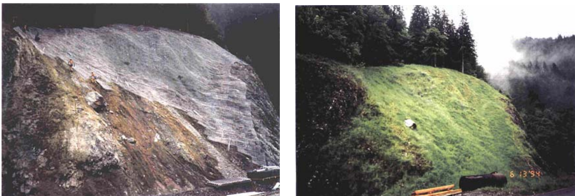
Figure 9. A rockslide before (on the left), which is partly covered with the lattice, and after (on the right) the stabilization with the "Krismer-Gitter" and the vegetation 3 months later
